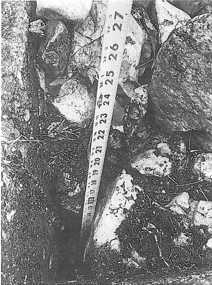
Figure 3 - Void next to trough right training wall 25" deep
